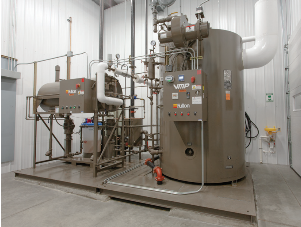
▲ The boiler room at Green Field Farms dairy features a Fulton VMP-100 boiler and accessories delivered as part of a fully-engineered, pre-piped, skid-mounted system.
