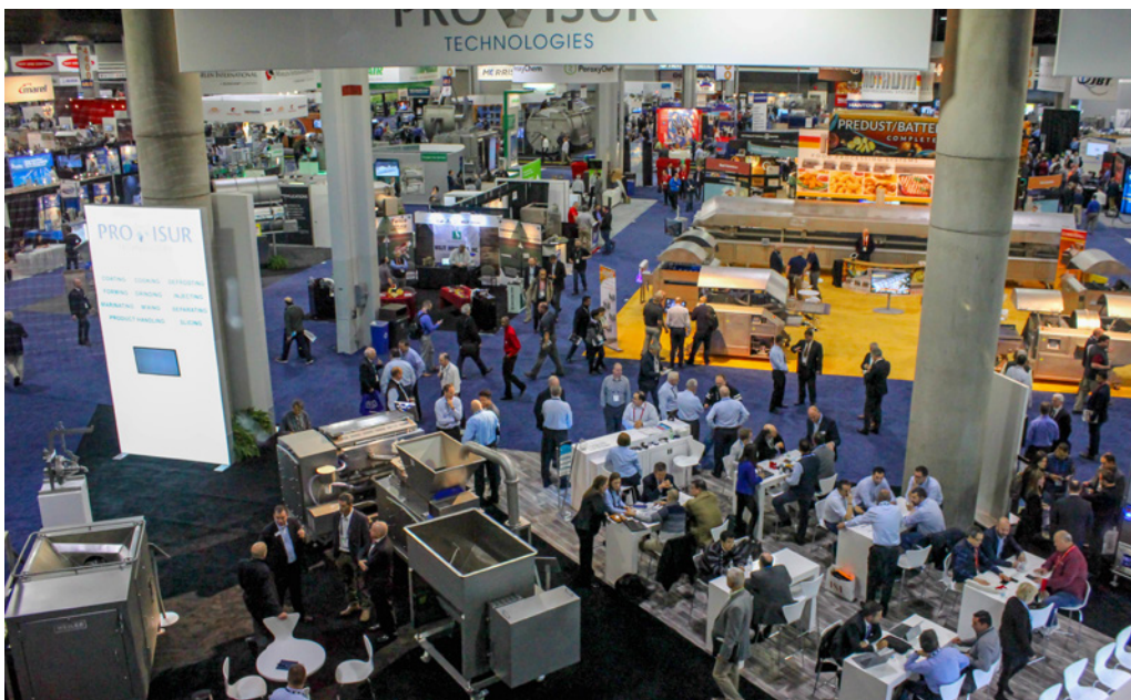
▼ One of the GWCC's twelve vast exhibit halls that is heated by six dual-fuel VTG boilers.
